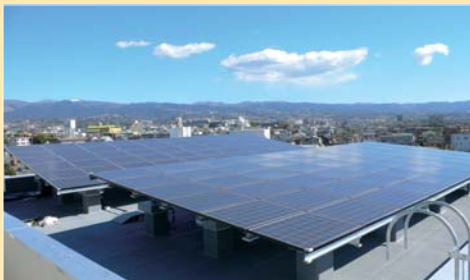
Photovoltaic power generation system
